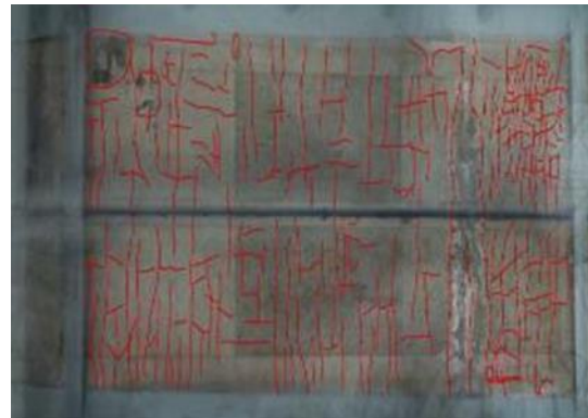
Figure 4. Created crack damages map.
